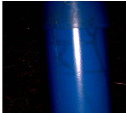
Leak causes no action
